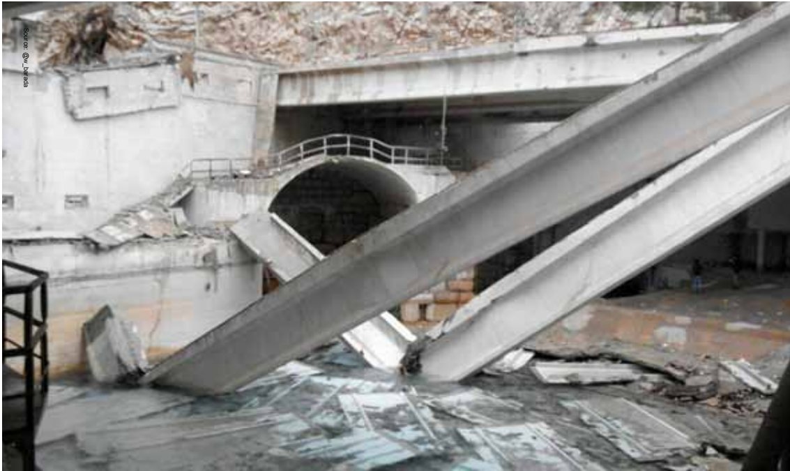
The damaged Wadi Barada water facility.
