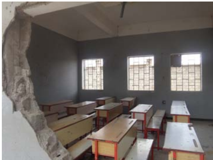
View of destroyed exterior of Asma'a bint Abi Bakr School in Al-Mansuriyah District, Hudaydah Governorate after August 2015 airstrike
