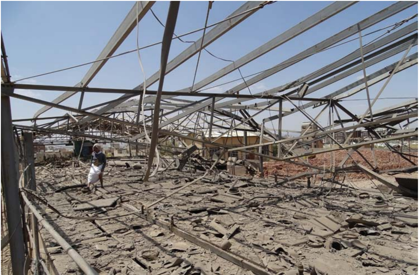
Man walks through rubble after September 2016 airstrike on Al-Senidar Factory Complex in Bani Al-Harith District, Amanat Al-Asimah Governorate.
